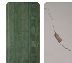
Walls - Cracks / Tears
