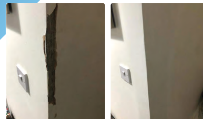
Corner of wall caught on delivery. Damaged area was cut out and re-skimmed to be even with the rest of the wall, and then repainted. Customer happy with the very quick turnaround.
