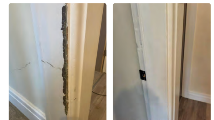
Door frame heavily damaged from delivery. Sanded the area, used wood-based filler where necessary, and finally repainted to match. Customer completely satisfied with repair.
